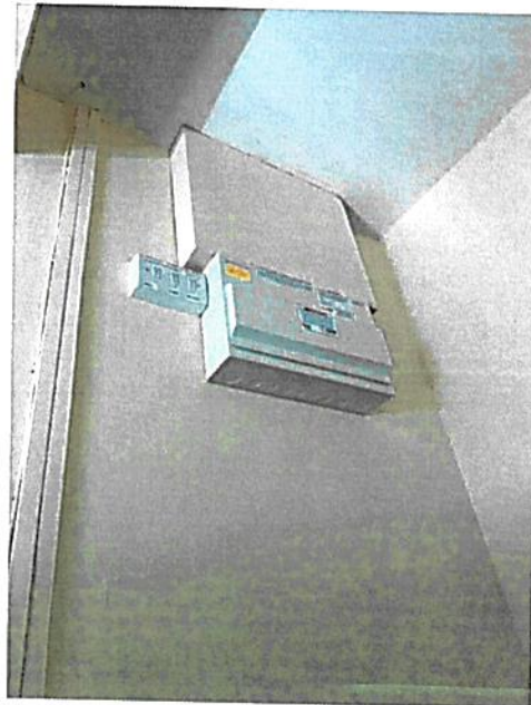
Electrical fuse board
