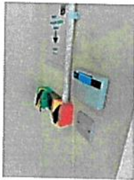
Call points covered with hazard tape
