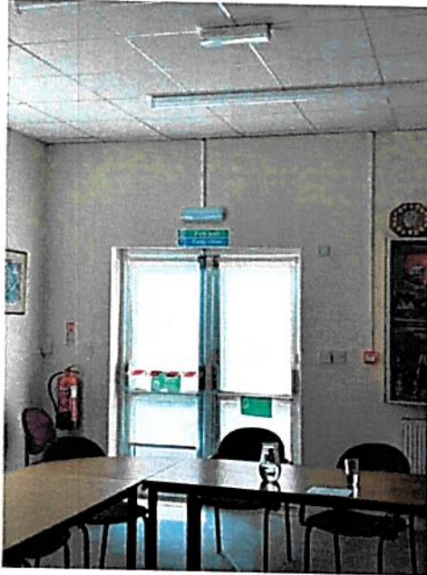
Fire exit door broken
