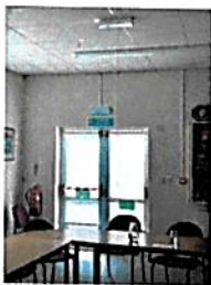
Fire exit door broken
