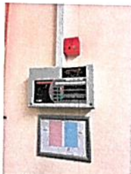
Fire alarm panel free from faults
