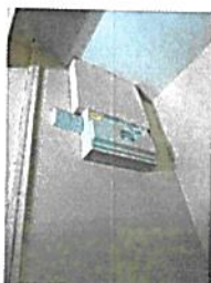
Electrical fuse board
