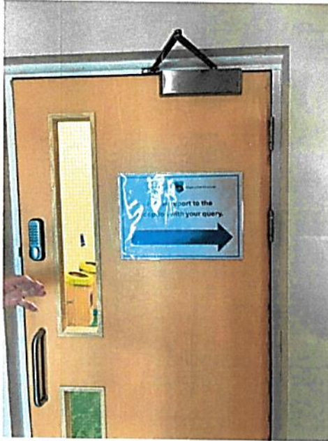
Fire exit door no signage on keep clear
